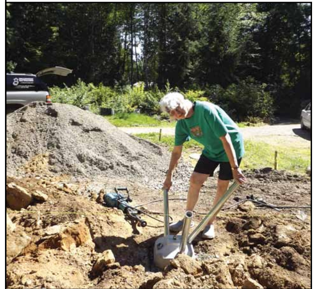
Sue Mitchell demonstrates how to drive in the steel pins that will create her home's foundation using the Pin Foundation method. Low impact construction techniques, such as the Pin Foundation method, have been gaining popularity in new construction and renovation projects throughout the Pacific Northwest.
