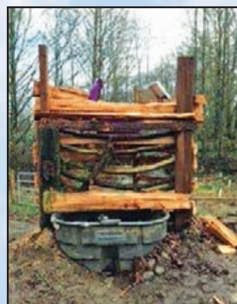
The landowner built a frame around his newly installed solar water pump to keep his cows from ruining it.
